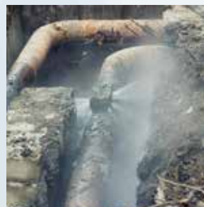
Cities lose 50% water due to leaking infrastructure
